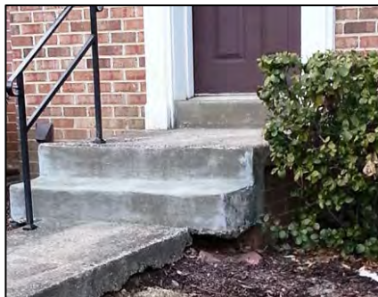
Erosion underneath steps needs to be addressed.
