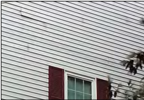
Siding needs to be repaired!
