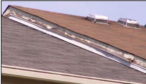
Rake board needs attention!
