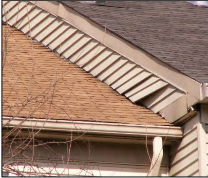
Upper story siding has come loose!
