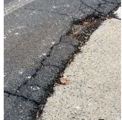
Street deterioration in Lafayette Village – soon to be milled and repaved!
