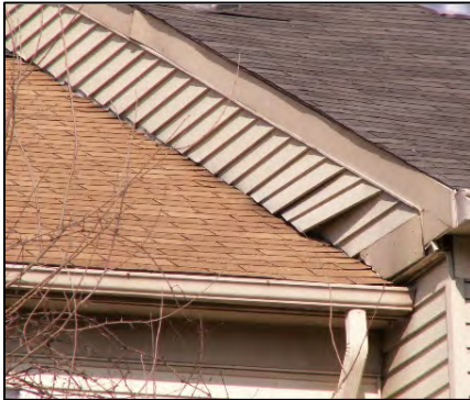
Upper story siding has come loose!
