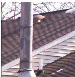
Chimney starting to corrode and rust!
