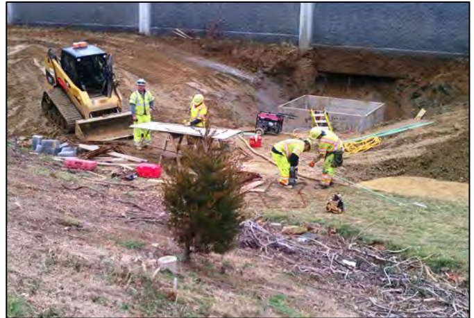
The new drain is visible in the back of this photo by the sound barrier.
