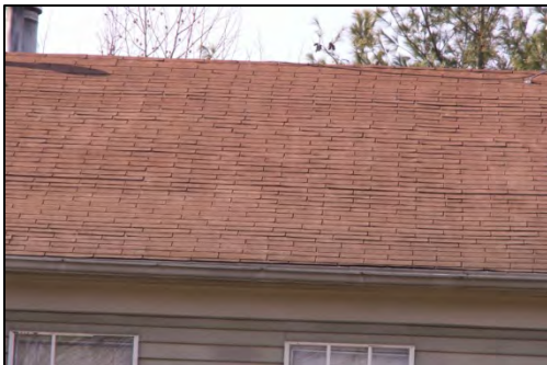
Roof looking to be replaced!
