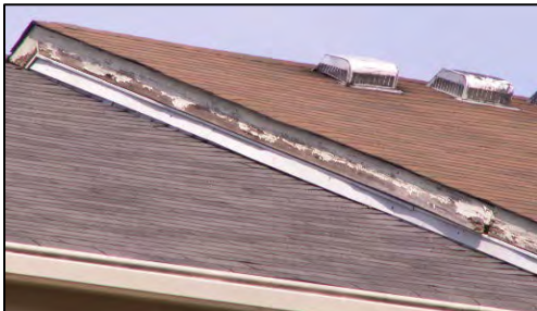
Rake board needs attention!
