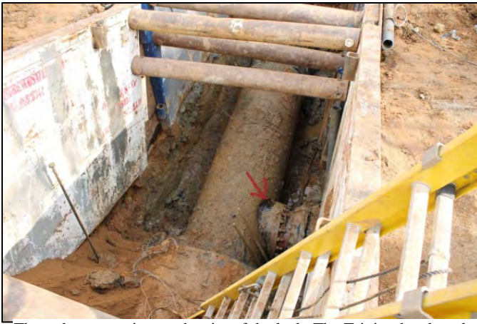
The red arrow points to the site of the leak. The T-joint developed a leak and needed to be replaced.
