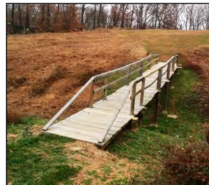
Meadows bridge after repairs. Note that Dominion mowed the meadows, which it does every 5 years.
