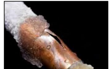
Burst water pipe
